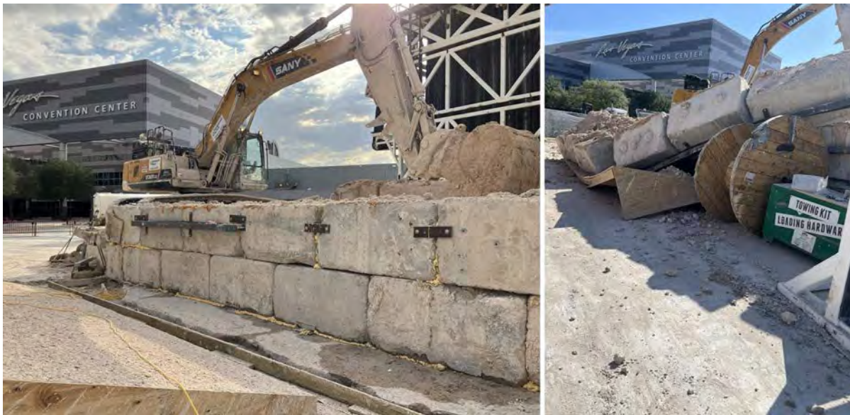
The collapsed muck bin, before (left) and after.
